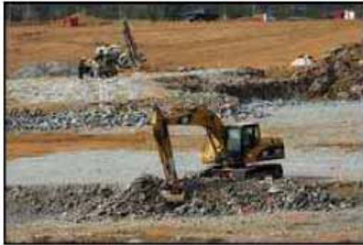
The Indian Lake Village project continues as construction crews clear a pad for a stadium-seating movie theater. LAVONDIA MAJORS / THE TENNESSEAN
